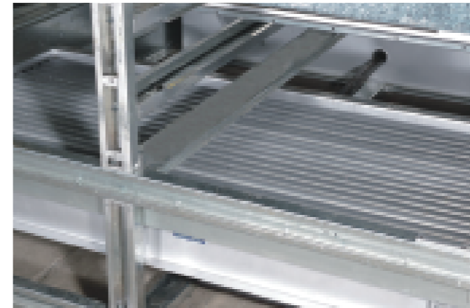
导热油加热 Thermo-oil heating
